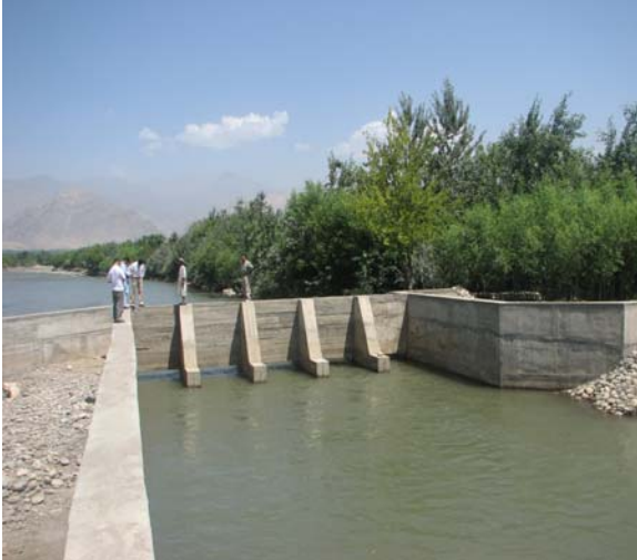
An irrigation intake, being built under the World Bank financed project in Kapisa Province.
