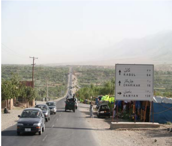
A view of Kabul - Salang highway, being rehabilitated under the World Bank financed project.
