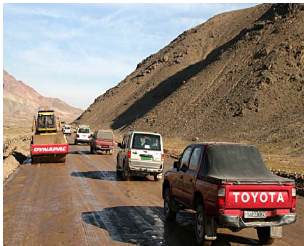
A view of Taloqan-Keshim road, under rehabilitation through the World Bank-financed Transport Project.
