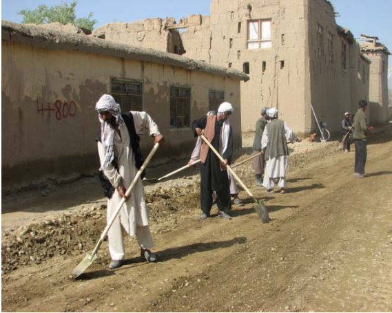
Locals work to rehabilitate a road under the NEEPRA project in Bagram district of Parwan Province.
