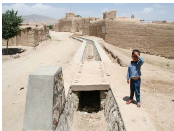
A cross drainage structure and a culvert have been built under the National Solidarity Program in a village in Ghazni Province.
