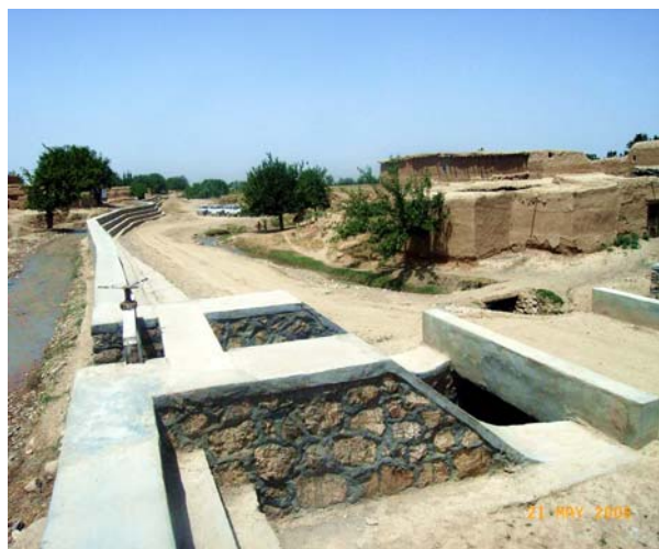
An irrigation in-take, being built under the World Bank-financed Irrigation Rehabilitation Project, in Jalalabad city.
