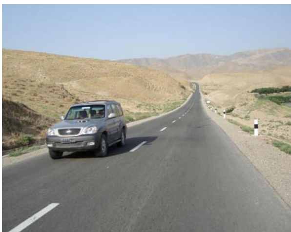
A view of Kunduz-Taloqan road, being rehabilitated under the World Bank-financed Transport Project.
