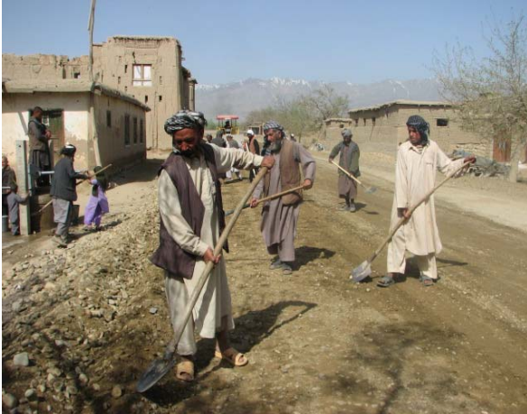
Locals work to rehabilitate a road under the NEEPRA project in Bagram district of Parwan Province.
