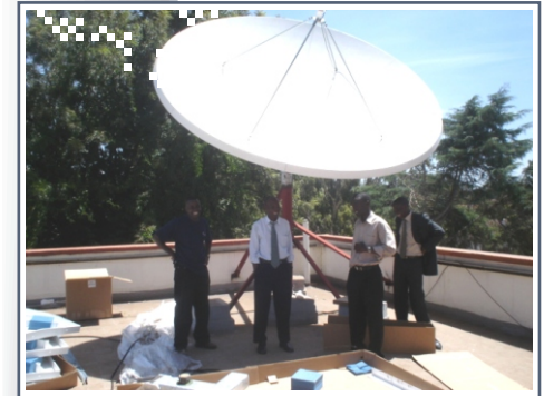
The VSAT being installed at the AVU Headquarters in Nairobi, Kenya
