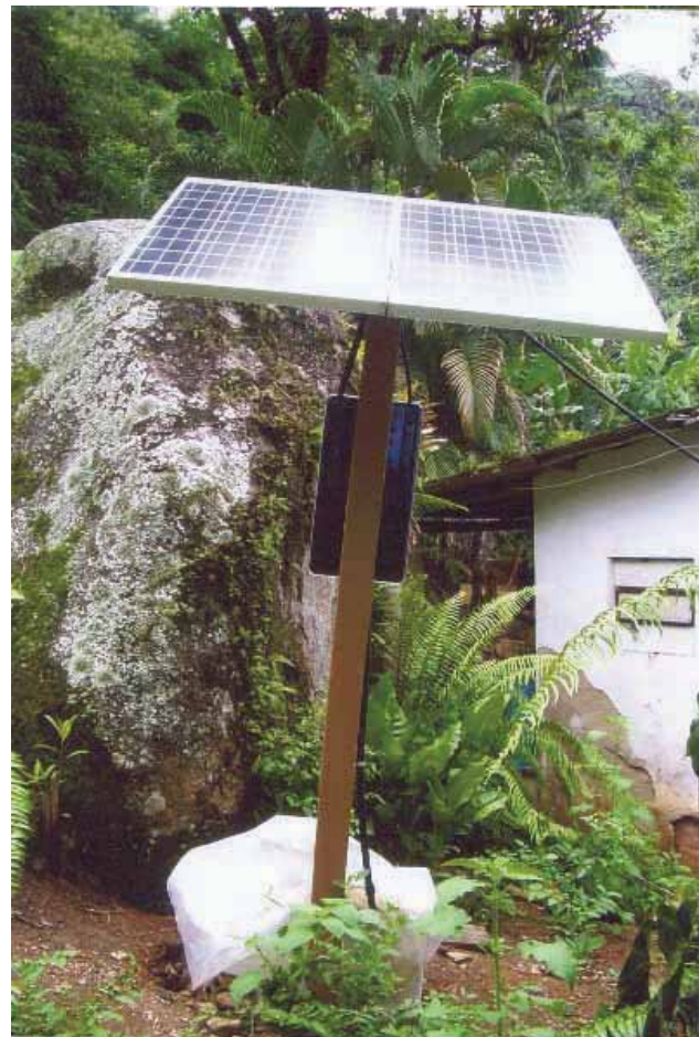
Solar home system, Brazil (Innovation for Development and South–South Cooperation, IDEAAS)
