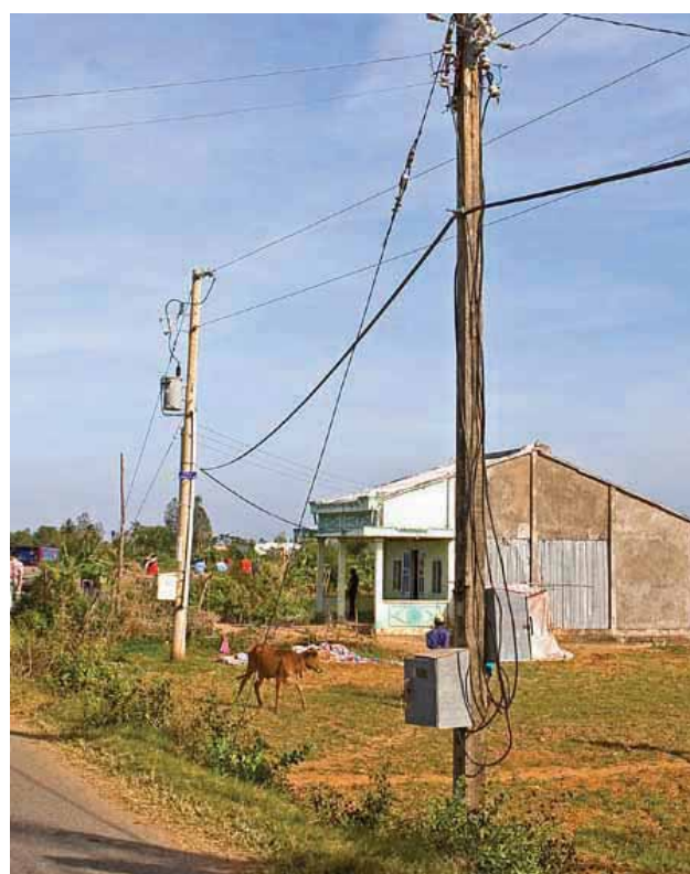
Grid rural electrification in Vietnam (World Bank, Hanoi)
