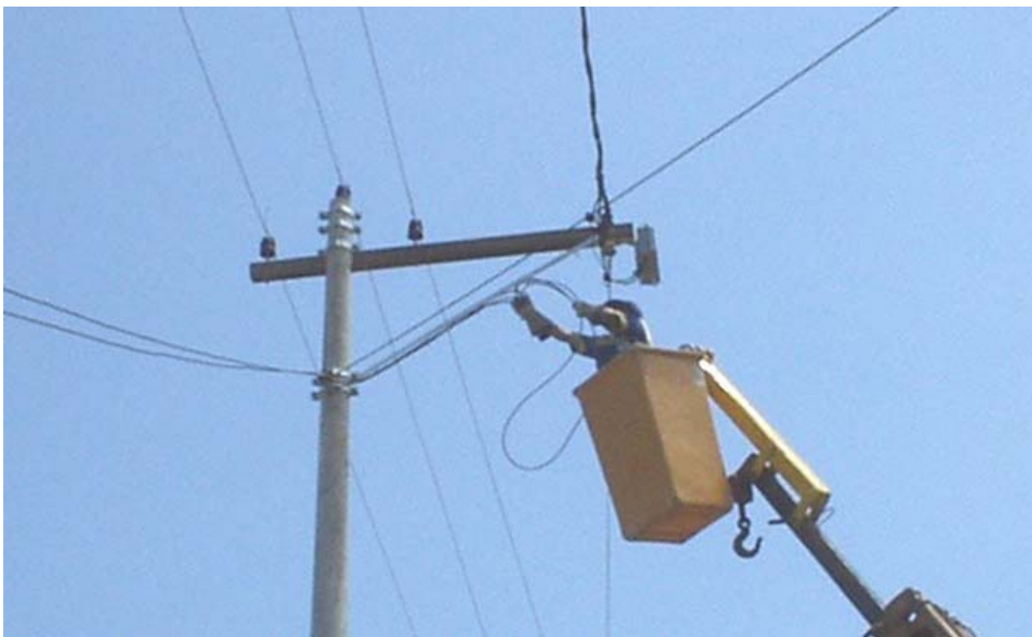
Figure 6: Shielded connections in MVD
