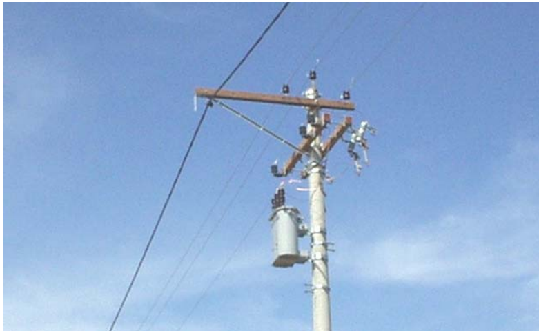
Figure 4: Low capacity single phase medium-voltage to low-voltage transformer
