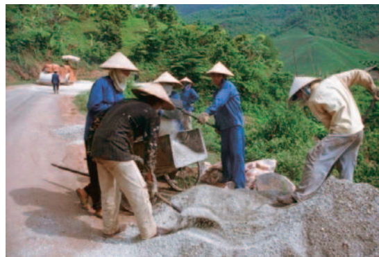
Construction crew upgrading the road between Lai Chau and Lao Cai towns, northern Vietnam, Photographer: Tran Thi Hoa, 2002.
