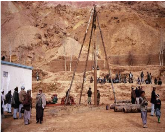
A well is dug as part of a community project to improve the drinking water supply in Sighan District, Bamayan province. The project was supported by Afghanistan's National Solidarity Program which is funded primarily by the World Bank.
