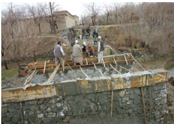
A bridge is built in Jabel Seraj District, Parwan Province with financing support from the World Bank National Emergency Employment Program for Rural Access
