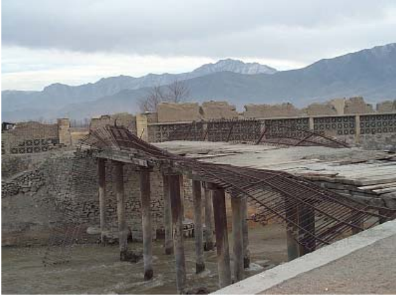
A crumbling Bridge in Logar province
