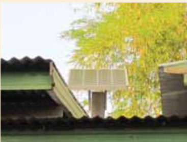
Mrs. Tim's 50w solar panel.
