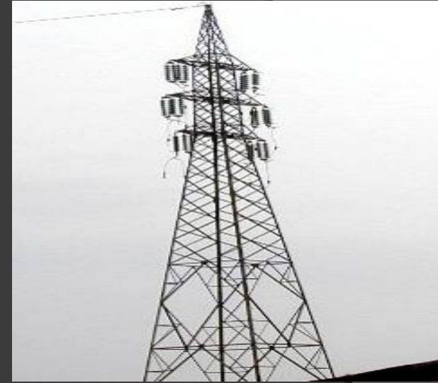
Towers - no conductors
