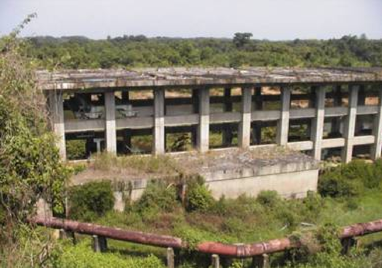
Mount Coffee Hydro Plant
