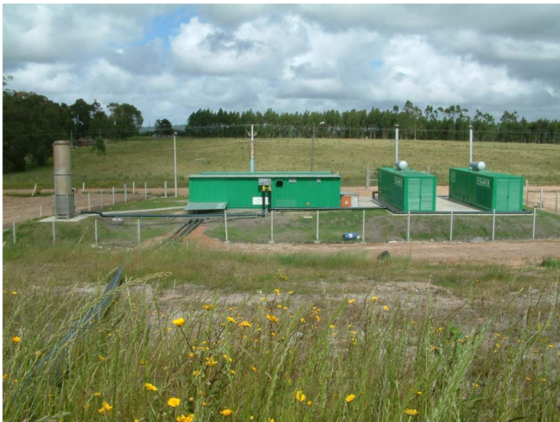
Figure 3. Landfill-gas-to-energy plant in Las Rosas landfill
