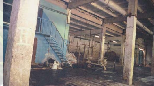
Storage space at Belon Tannery used for excess chemicals and wet skins. The floor is wet with Cr+4 contaminated water.
