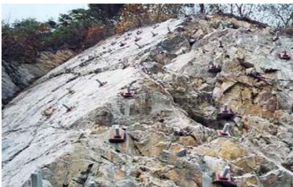
Figure 4. Rock bolts and anchors, Hongchon Street No. 36, Gangwondo Province, South Korea
