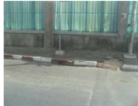
Posts in the middle of the road
