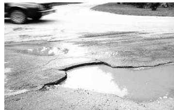
Condition 4: Safety Hazard
