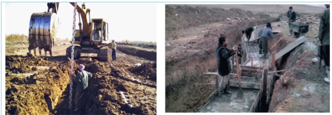
Digging of a canal near Baghdad and construction of a water conduit near Sulaymaniyah (Northern Iraq) as part of the WB Emergency Community Infrastructure Project (February 2006)
