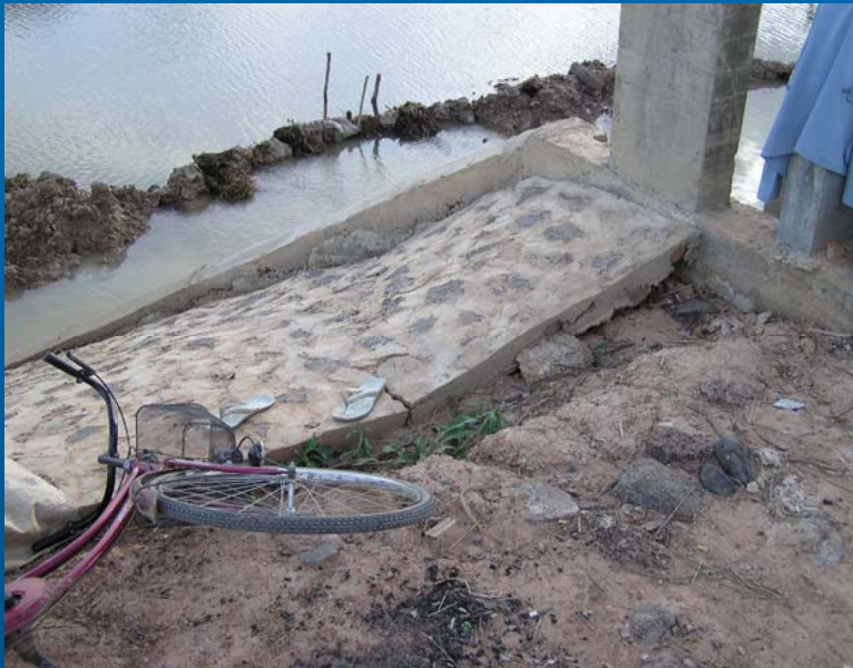
Settlement and cracking of rip-rap adjacent to main sluice gate structure
