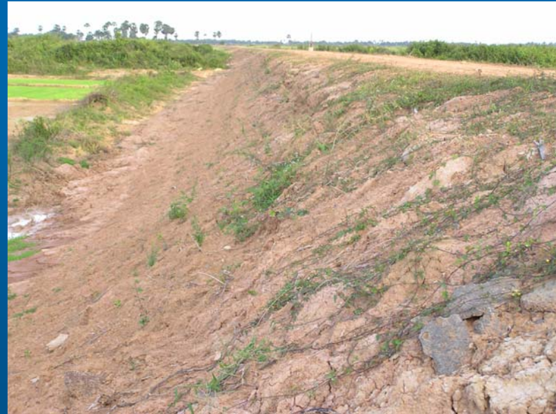
Earth bund already showing erosion
