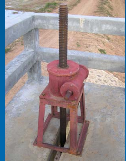
Sluice-gate mechanism starting to rust
