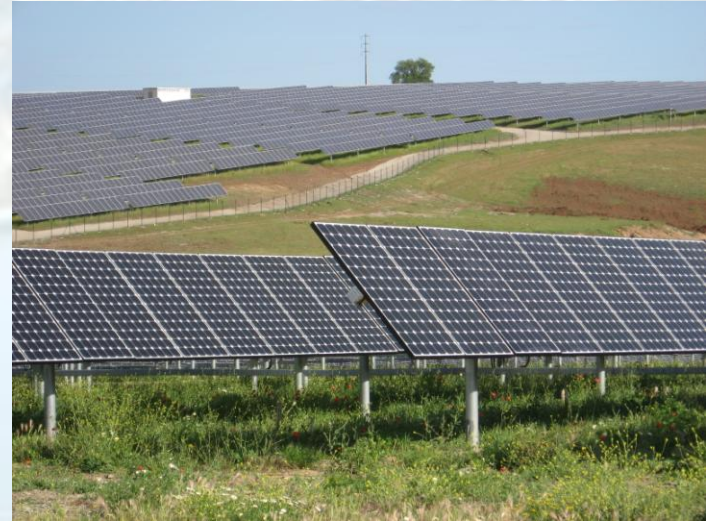
Solar PV – Serpa, Portugal
