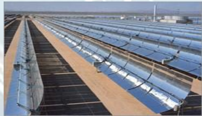
Concentrating Solar Power (CSP) Parabolic Troughs – Nevada USA
